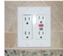
Example of ↑ GFI receptacle
